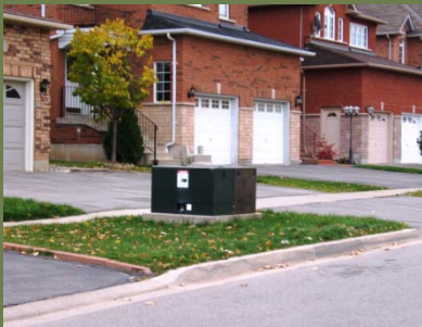
Pad mounted transformer
