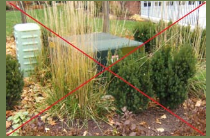
Obstruction around a transformer
