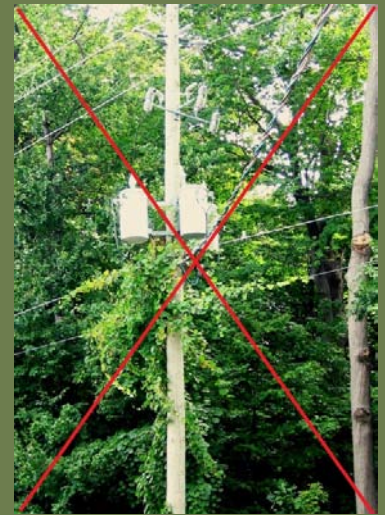
Pole growth contacting electrical equipment & powerlines
