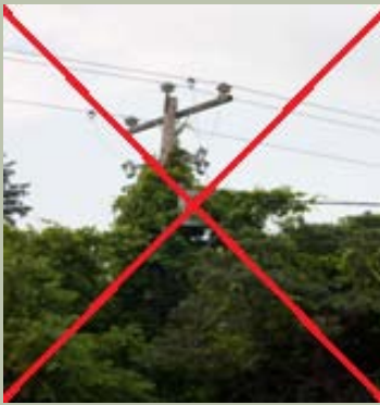
OVERGROWN VINES AROUND ELECTRICAL EQUIPMENT
